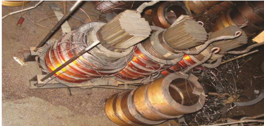
Fig. Failure due to paper block shrinkage
