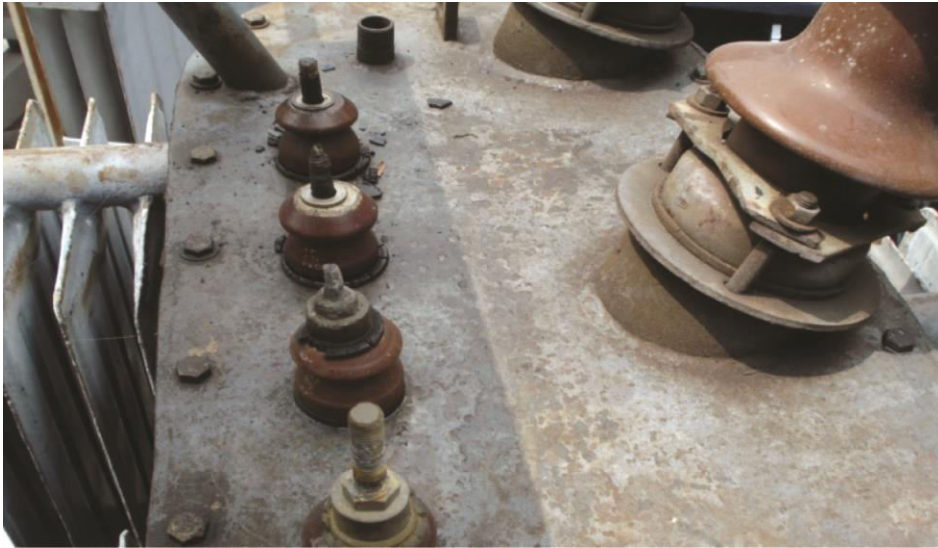
Fig. : Improper joint
