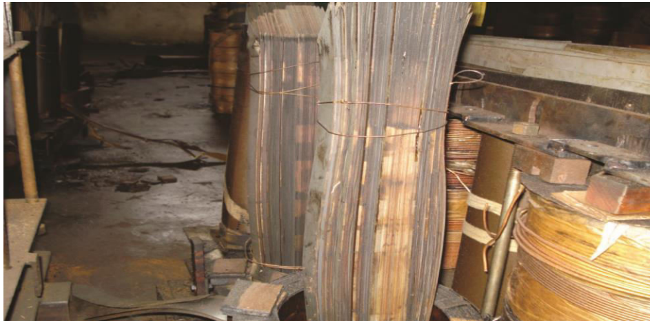
Fig.: Core insulation failure
